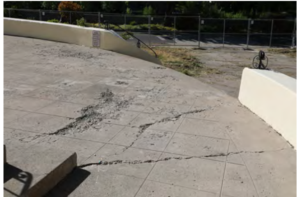
Figure 04: Significant spalling of the concrete of the south entrance Terrace
