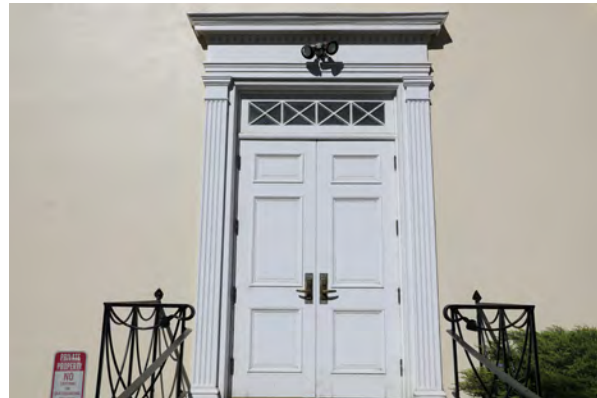
Figure 23: Exterior flood light at the East Entry
