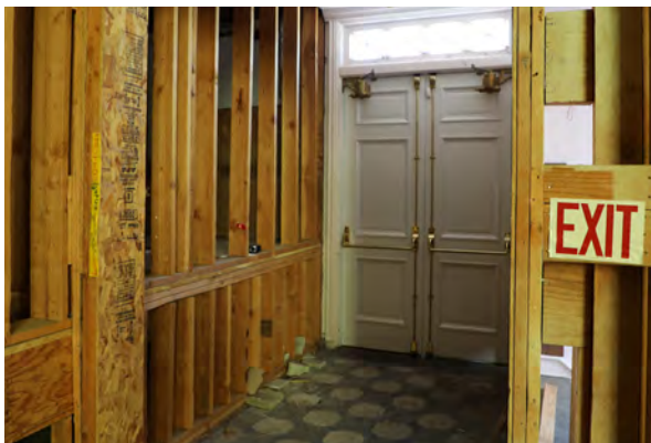
Figure 27: Unfinished construction at the East Entry (Room 109) showing rough opening and wall framing
