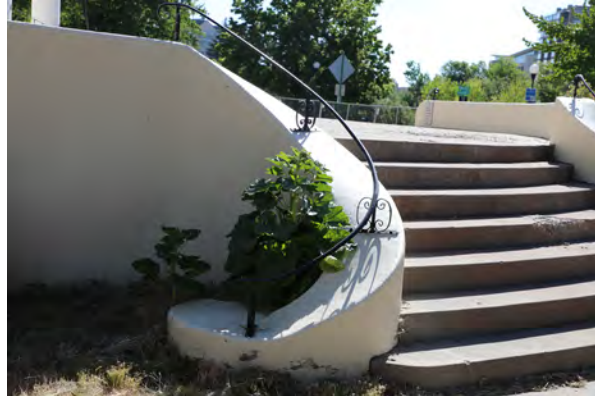
Figure 02: Non-compliant handrails at the southwest stair
