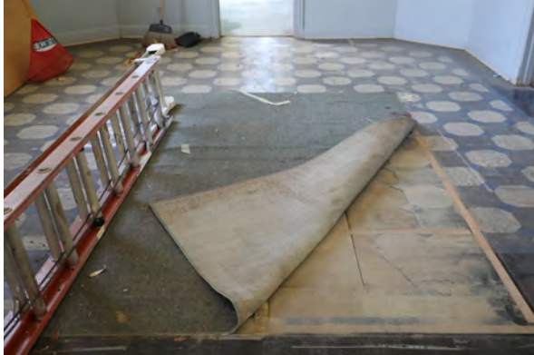
Figure 31: Fire damaged and missing vinyl tile under a temporary carpet section in the west Lobby (Room 115)
