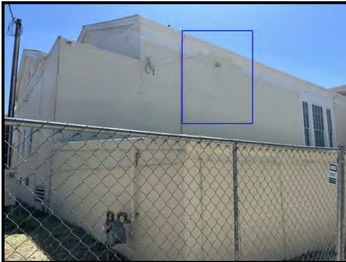
Figure 30 View of bubbling plastic membrane at the west exterior wall.
