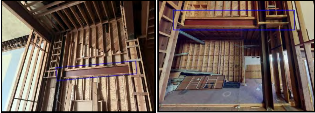
Figure 18 View of west (left) and east (right) steel framing above the stage.
