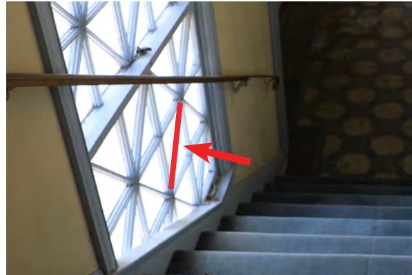
Figure 16: Missing interior muntin at Window 1-12
