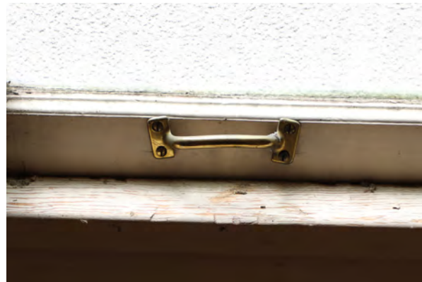
Figure 22: Damaged (bent) hardware at Window 2-04 in the Committee Room (Room 204)
