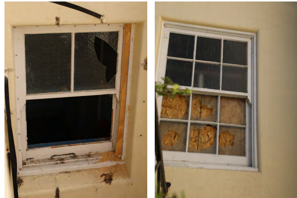
Figure 17: Damaged sash and broken or missing glazing at Windows 0-10 (left) and 1-10 (right)
