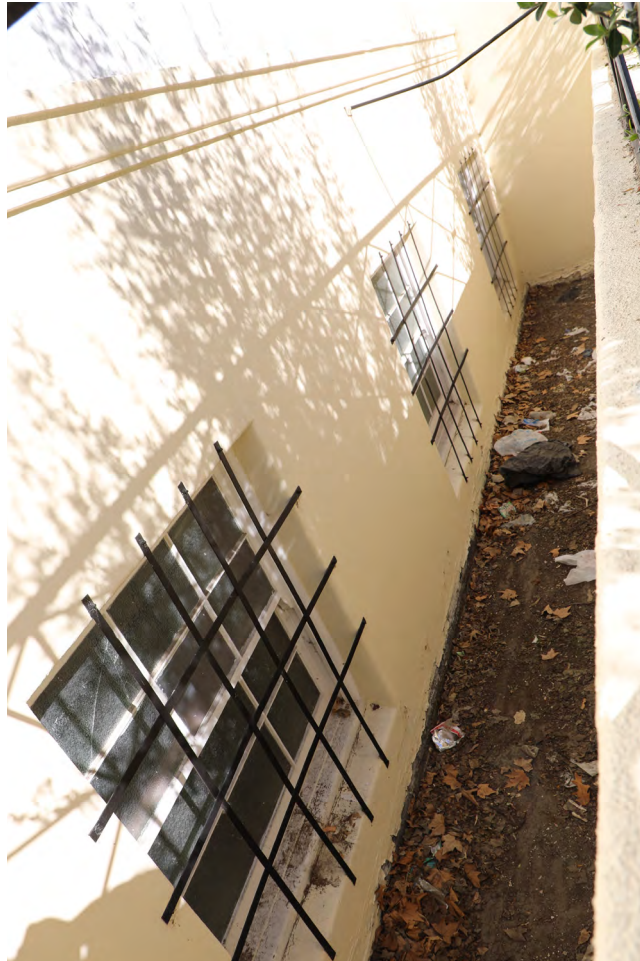
Figure 11 - View into areaway at basement windows along the east facade, view north (ARG, 2024)
