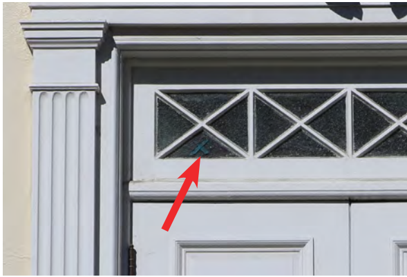
Figure 14: Cracked glazing at east entry transom
