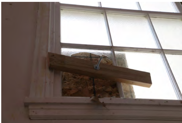
Figure 21: Broken glazing in bottom sash of Window 1-05 at the northern stairs (Room 008)
