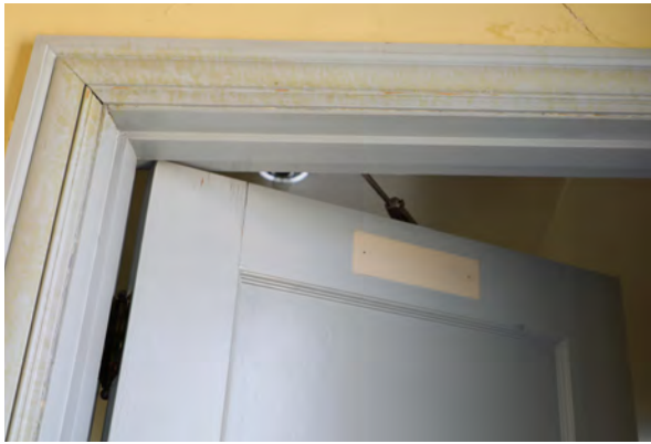
Figure 26: Missing paint at the top rail of the Men's Restroom (Room 105) door and yellow residue visible at the trim
