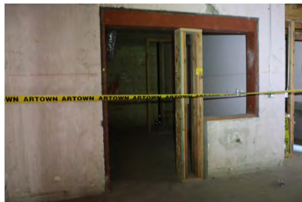
Figure 30: Unfinished openings in basement
