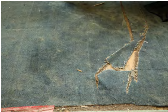
Figure 32: Damaged and worn broadloom carpet in Auditorium (Room 107)
