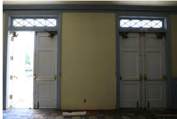
Figure 34: Missing wainscot between Door 1-14 and Door 1-15 in the Foyer (Room 101)
