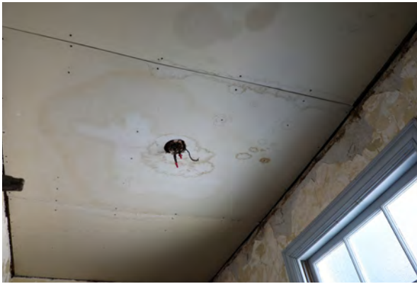
Figure 38: Moisture damage, unfinished drywall, and removed light fixture at ceiling of west Women's Restroom (Room 112)
