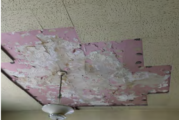
Figure 37: Missing acoustic tile and damaged historic finish at ceiling of the Literature Room (Room 114)
