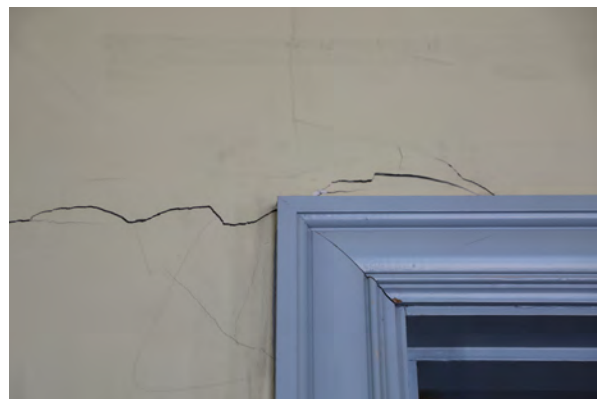
Figure 36: Significant cracking of plaster at cased opening on the north wall of west Lobby (Room 115)
