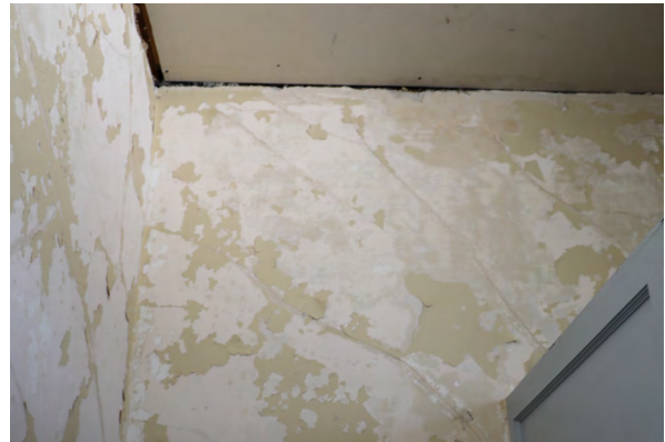
Figure 35: Severely damaged paint finish and plaster, possibly caused by ivy removal in the west Women's Restroom (Room 112)
