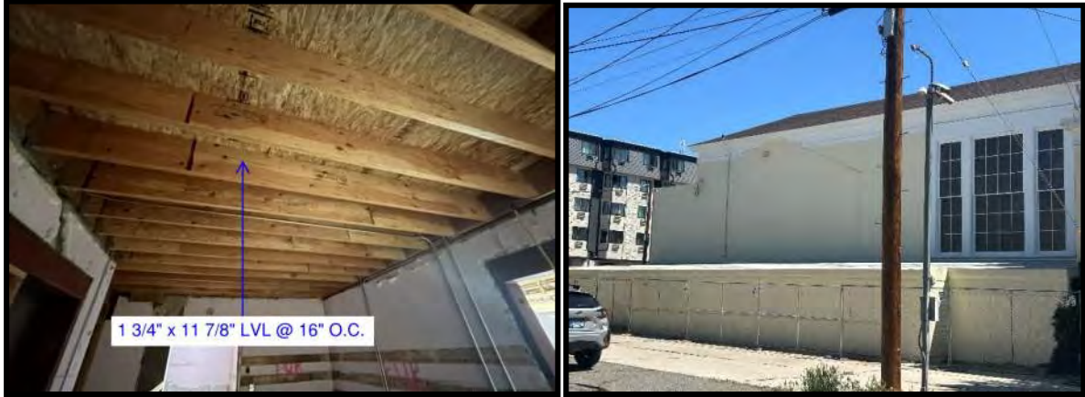
Figure 13 View of the 2002 first floor framing from the basement (left). View of the 2002 sleeper floor from the exterior of the building (right).
