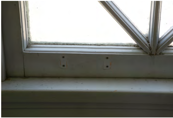
Figure 20: Missing hardware at bottom sash of Window 1-16 in the West Lobby (Room 115)
